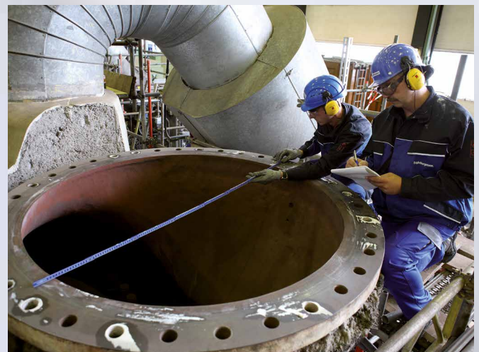
A flange is measured for the on-site production of a seal with 2,000 mm diameter.
